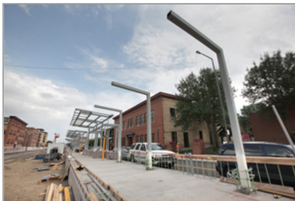
A Central Corridor LRT station was taking shape in August on University Avenue two blocks east of Raymond Avenue in St. Paul. The station is one of 53 sites designated as "transit improvement areas" and eligible for grant money to support development. (File photo: Bill Klotz)
