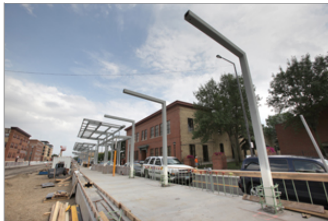
Central Corridor project workers are now building light rail transit stations at a number of the planned stops, including this one at Raymond Avenue. (Staff photo: Bill Klotz)
